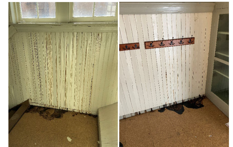
Figure 35 – Existing water damage inside the Princess Street Center
