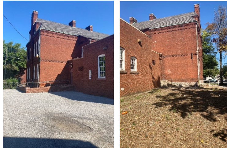
Figure 38 – Existing exterior repairs of the Princess Street Center
