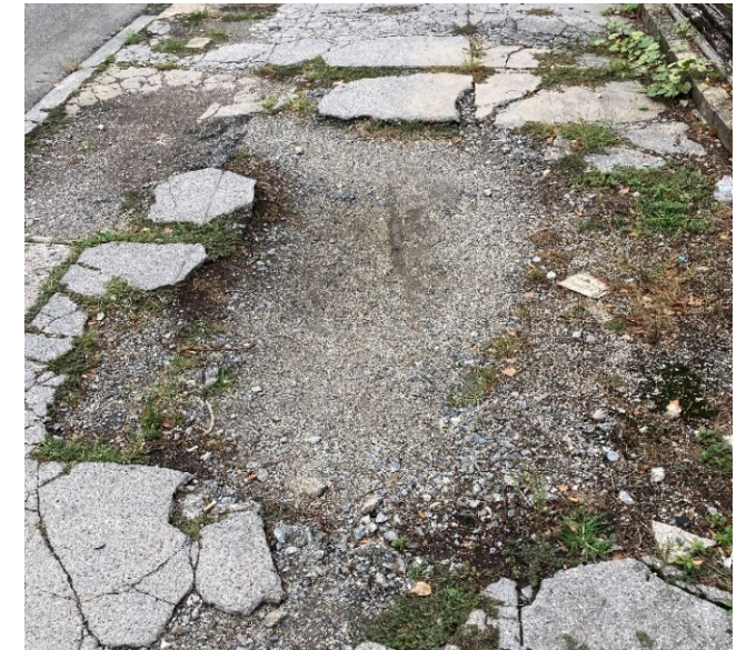
Figure 5 – Existing sidewalk conditions on Penn Street
